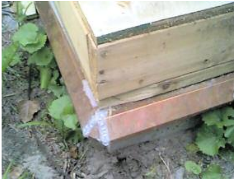
Figure D1.4 – Metal termite shield using copper metal on top of foundation wall. Copyright ©1998-2005, Urban Entomology Program, University of Toronto www.utoronto.ca/forest/termite/termite.htm
