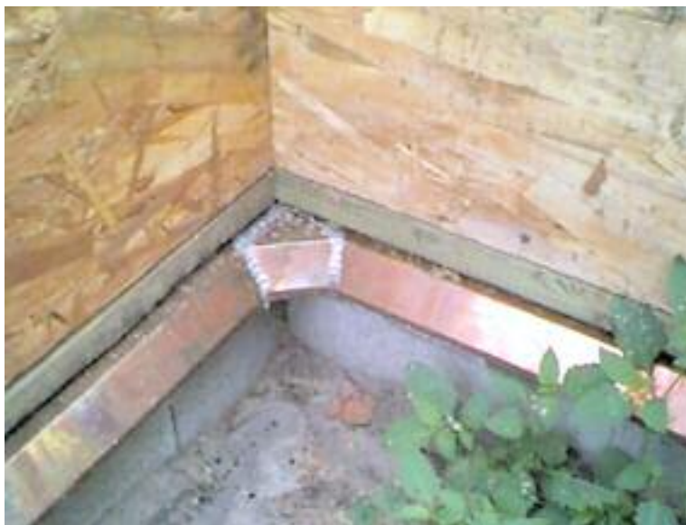
Figure D1.5 – Detail of metal shield at corner. Copyright ©1998-2005, Urban Entomology Program, University of Toronto www.utoronto.ca/forest/termite/termite.htm
