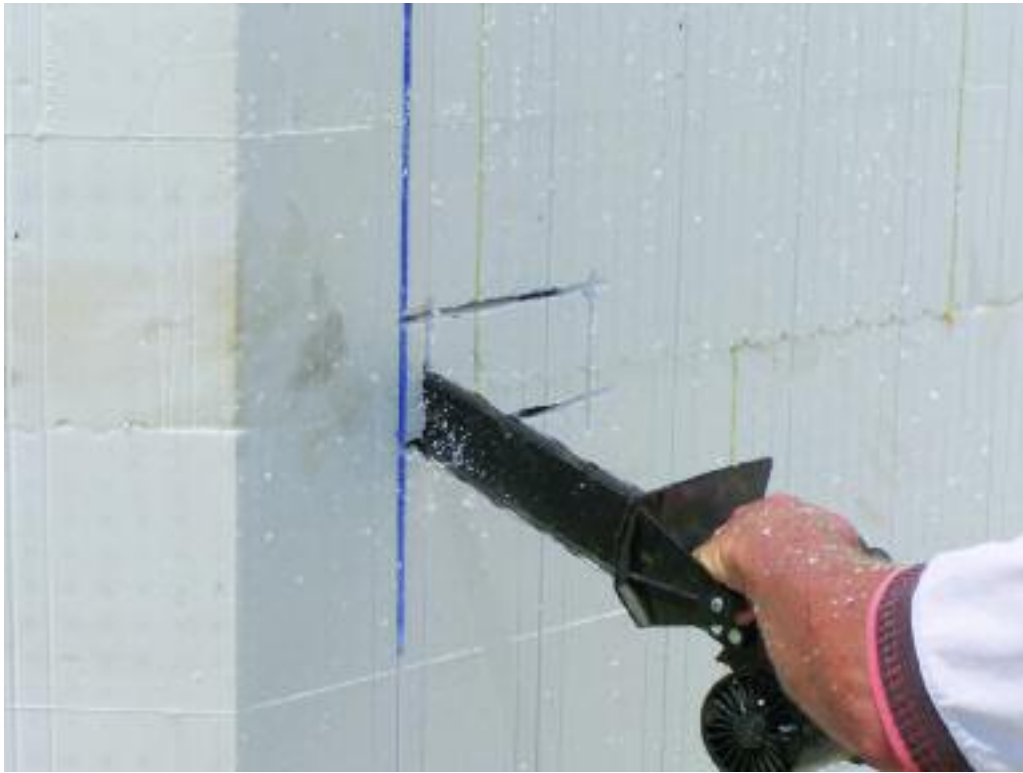
Figure E1.2 – Cutting a channel in the EPS panel using a chainsaw
